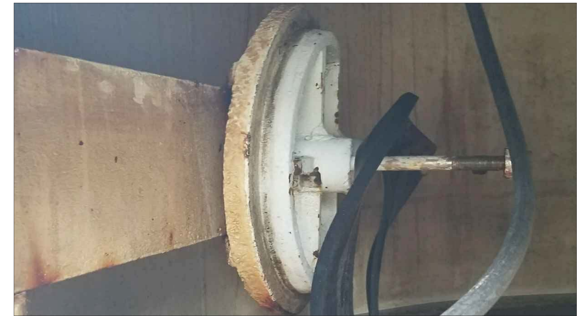
Figure 12. Interior Riser Access Way Repair minor corrosion on access way
