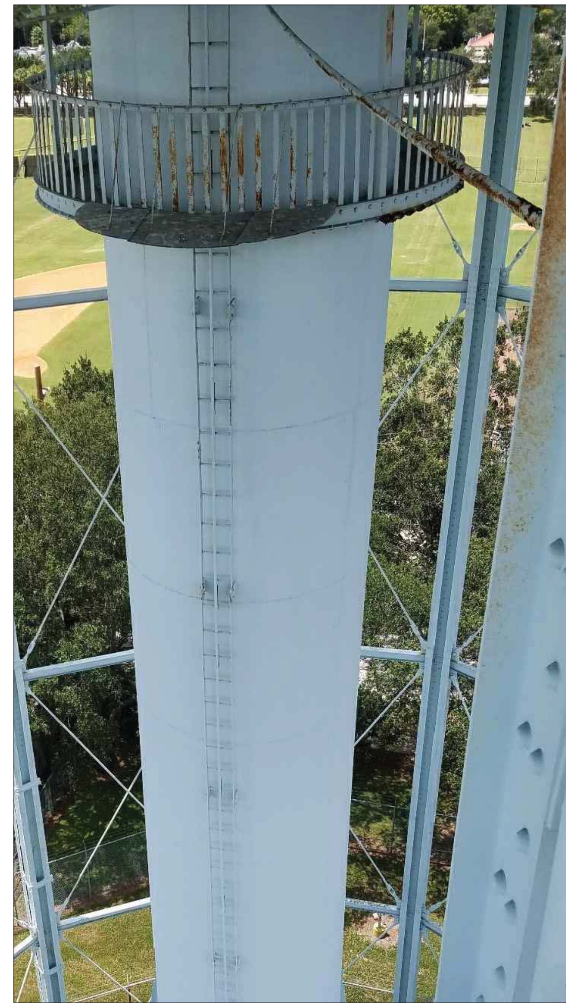
Figure 27. Exterior Inner Riser Ladder This ladder and associated platform was not inspected
