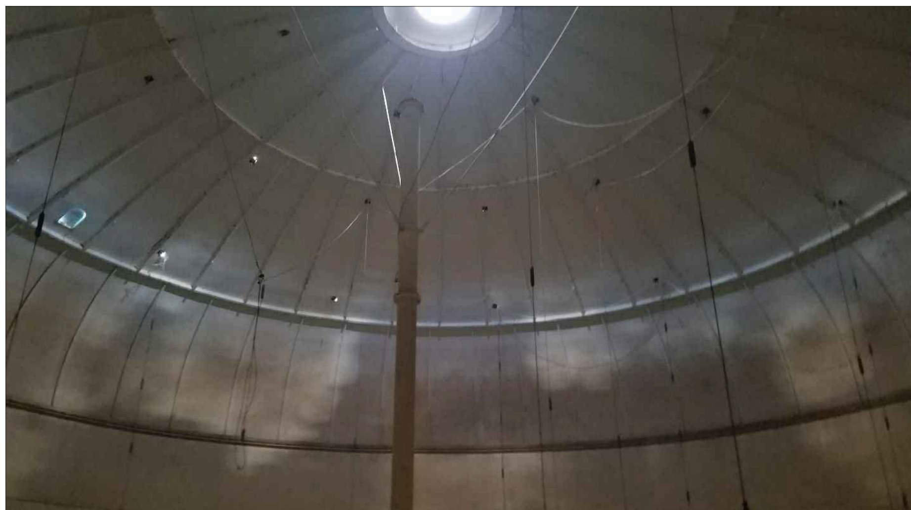
Figure 13. Interior Bowl Cathodic Projection System and Influent Pipe Provided for reference
