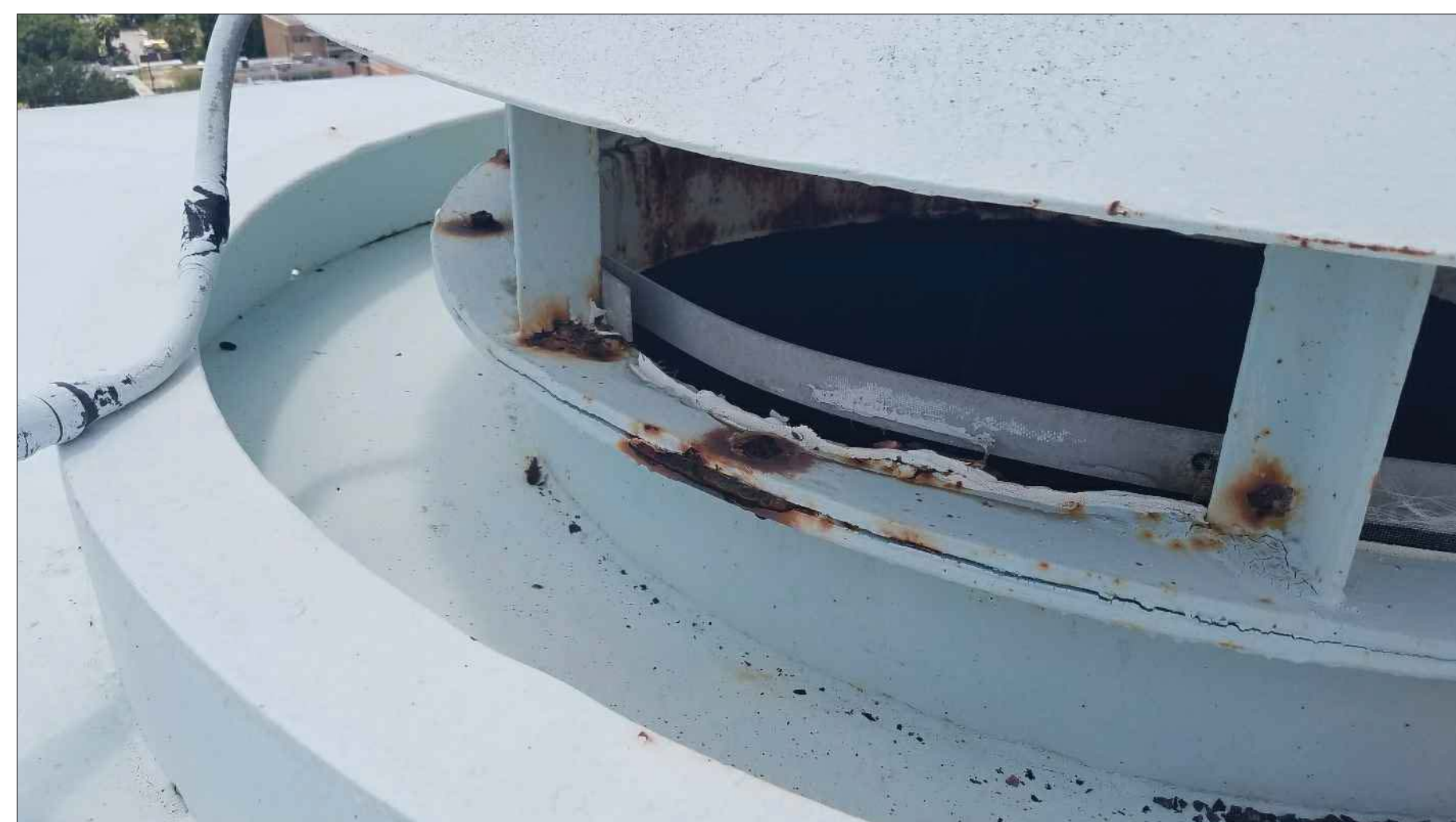
Figure 8. Top of Bowl Vent Repair corrosion at flange bolts and replace missing insect screen
