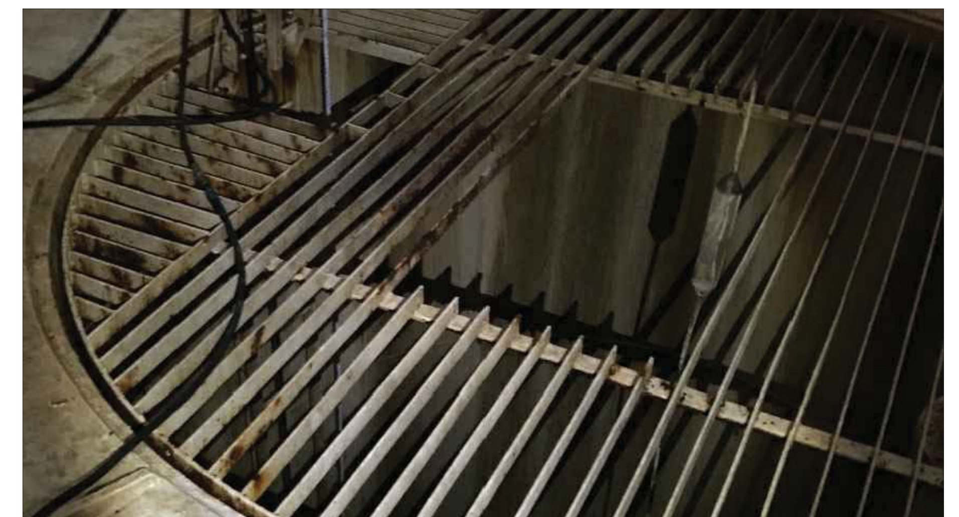
Figure 18. Grating at Top of Tank Riser Repair corrosion of grating
