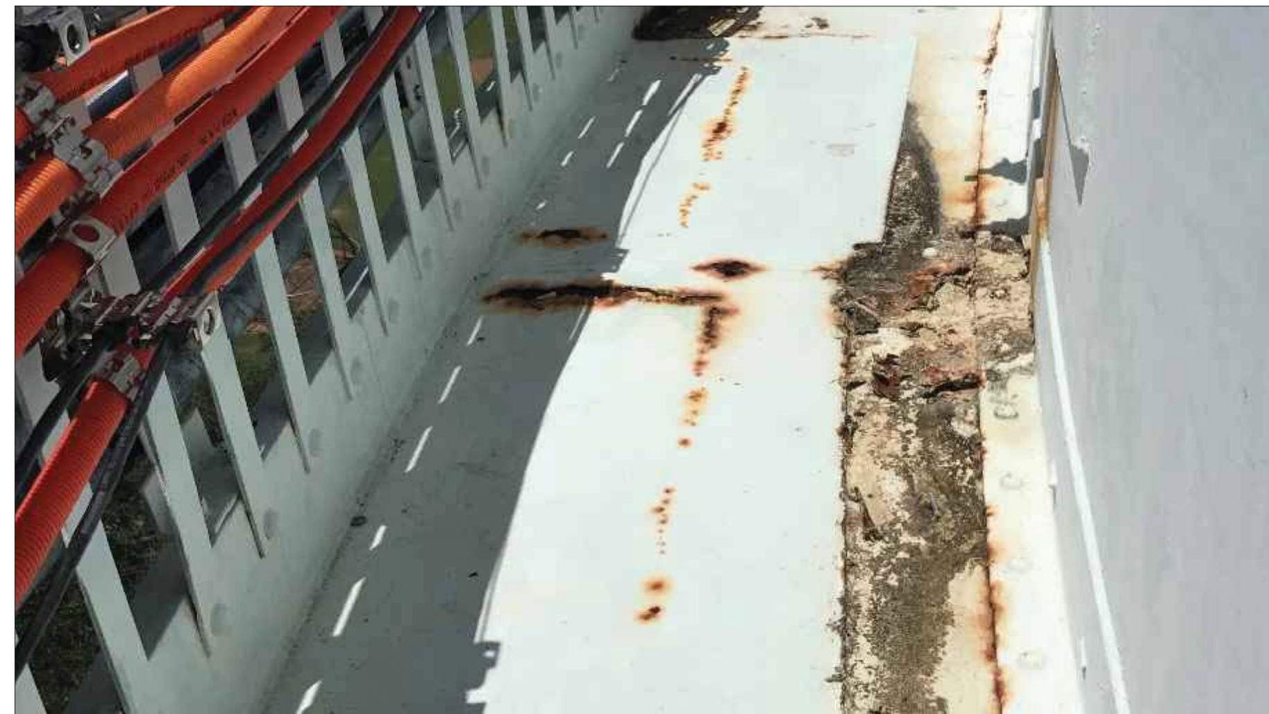
Figure 5. Exterior Bowl Platform Repair floor plate corrosion
