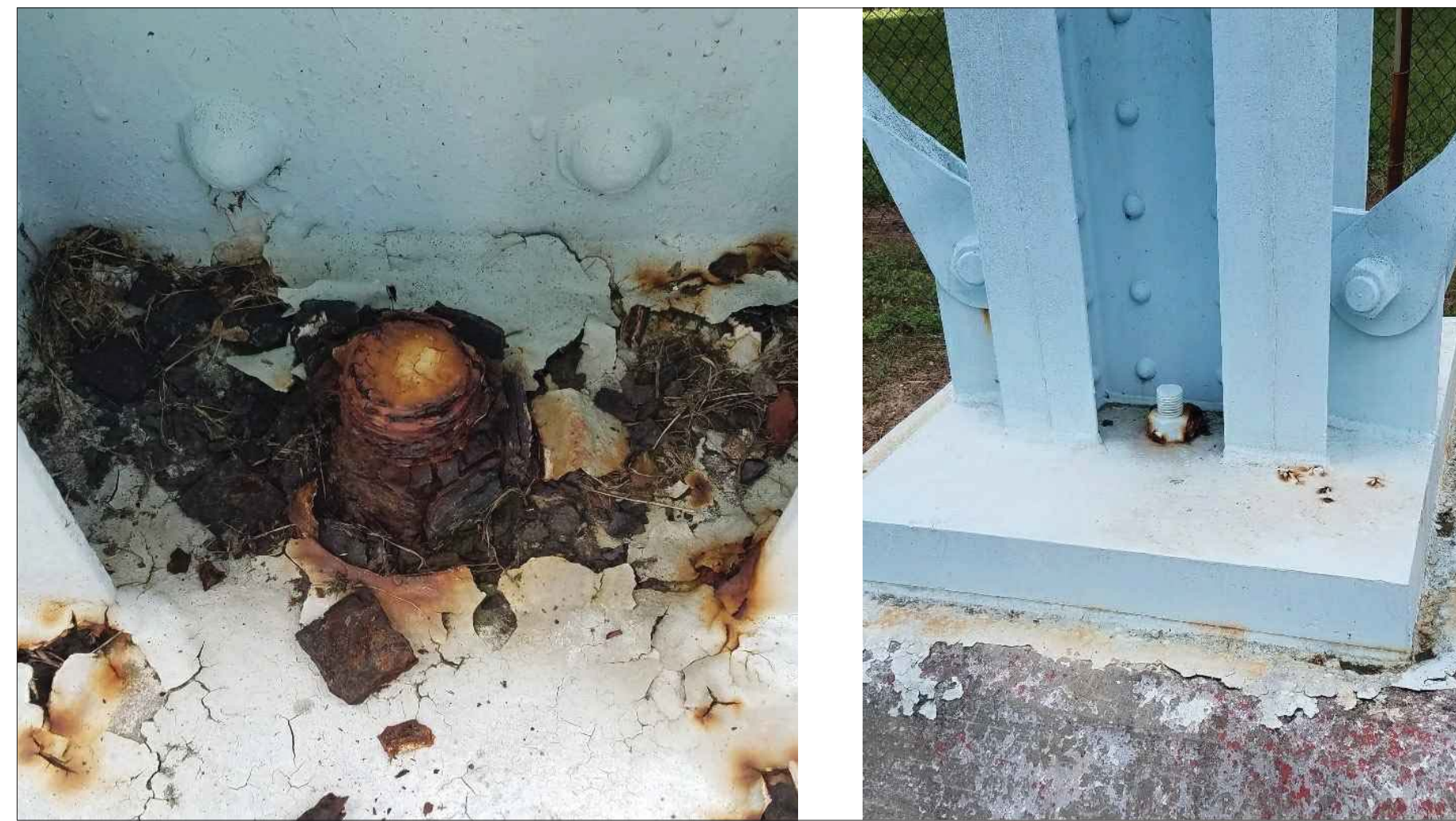
Figure 2. Column Anchor Bolt and Nut Repair corrosion on column anchor bolts and nuts.
