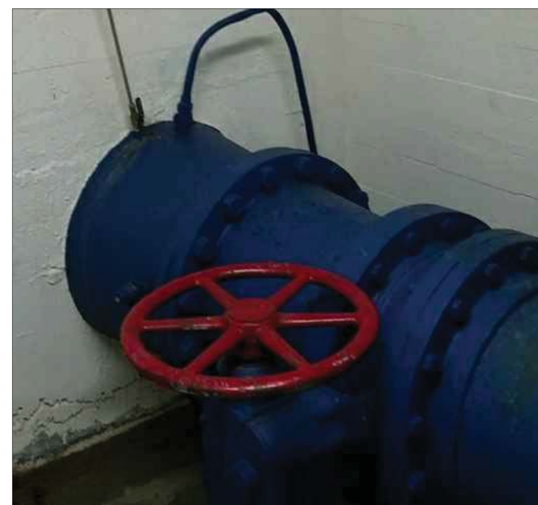
Figure 25a. Isolation Valves Remove and replace Isolation Valves
