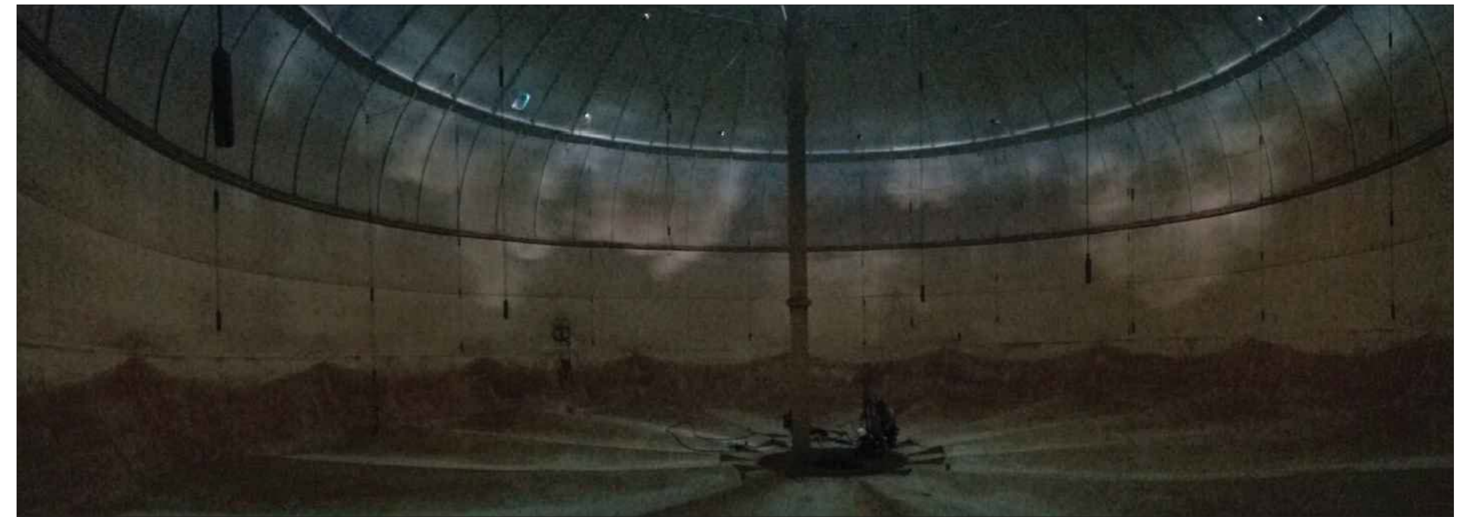
Figure 20. Interior Tank Bowl Provided for reference
