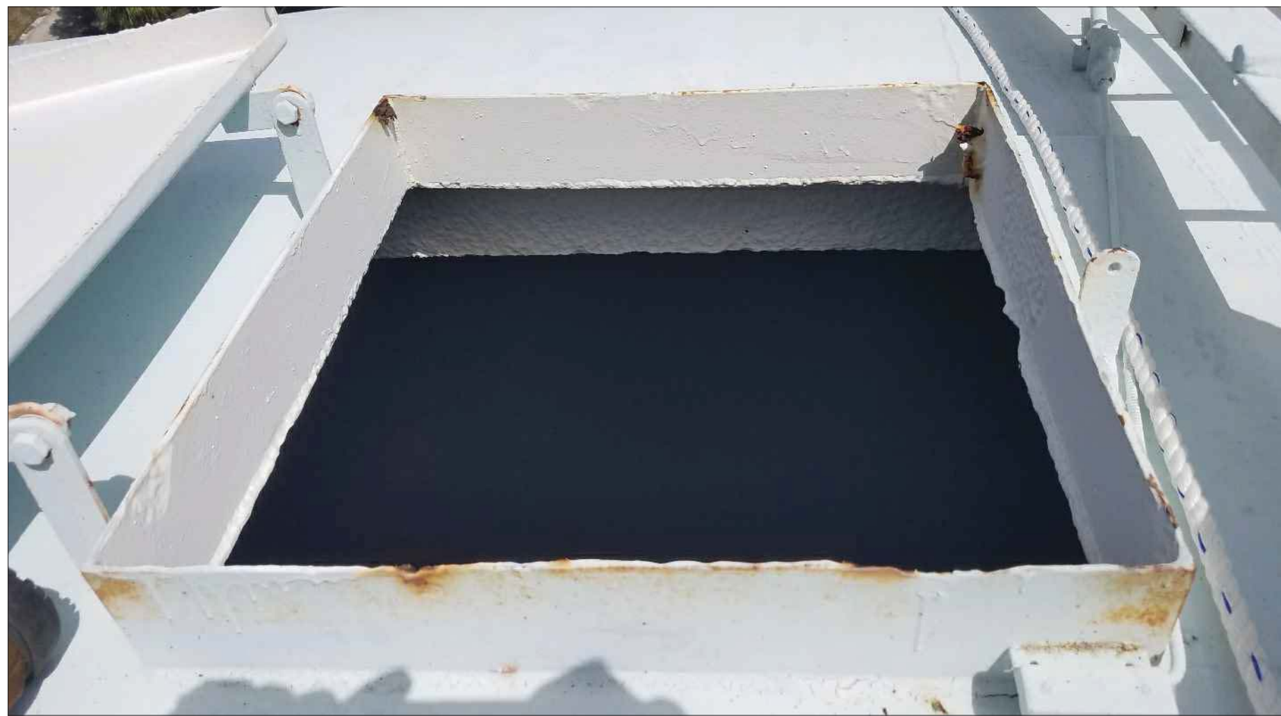
Figure 10. Top of Bowl Access Way Repair minor corrosion on access way
