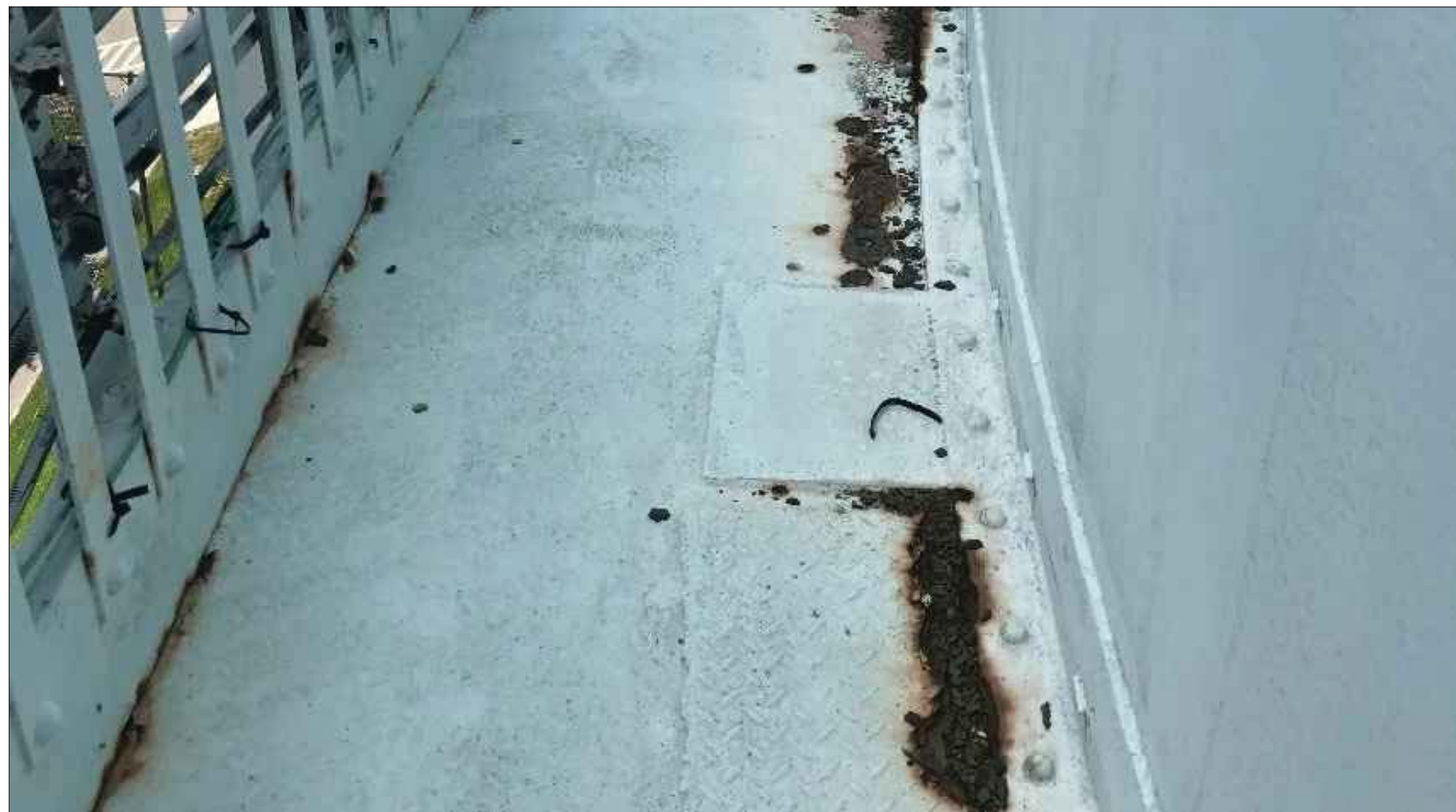
Figure 4. Exterior Bowl Platform Repair floor plate corrosion
