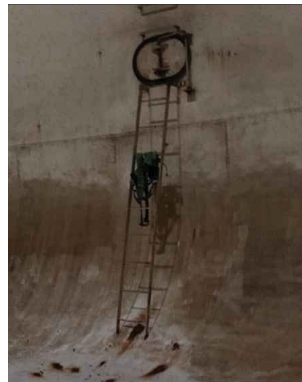
Figure 32. Interior Bowl Ladder Remove and replace interior ladder. Repair corrosion at ladder base and on tank interior.
