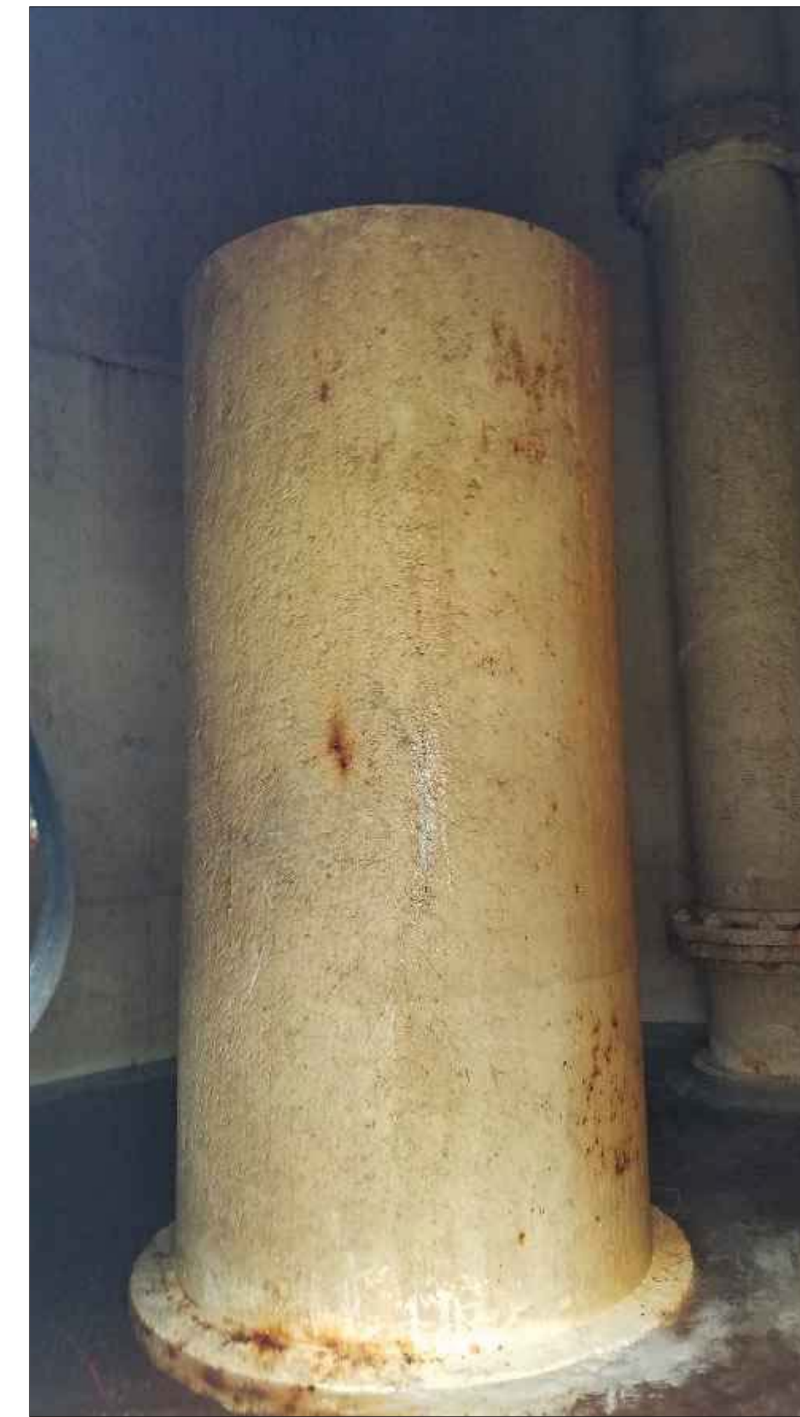
Figure 29. Tank Influent and Effluent Pipe Lines Repair minor corrosion on influent and effluent pipe lines
