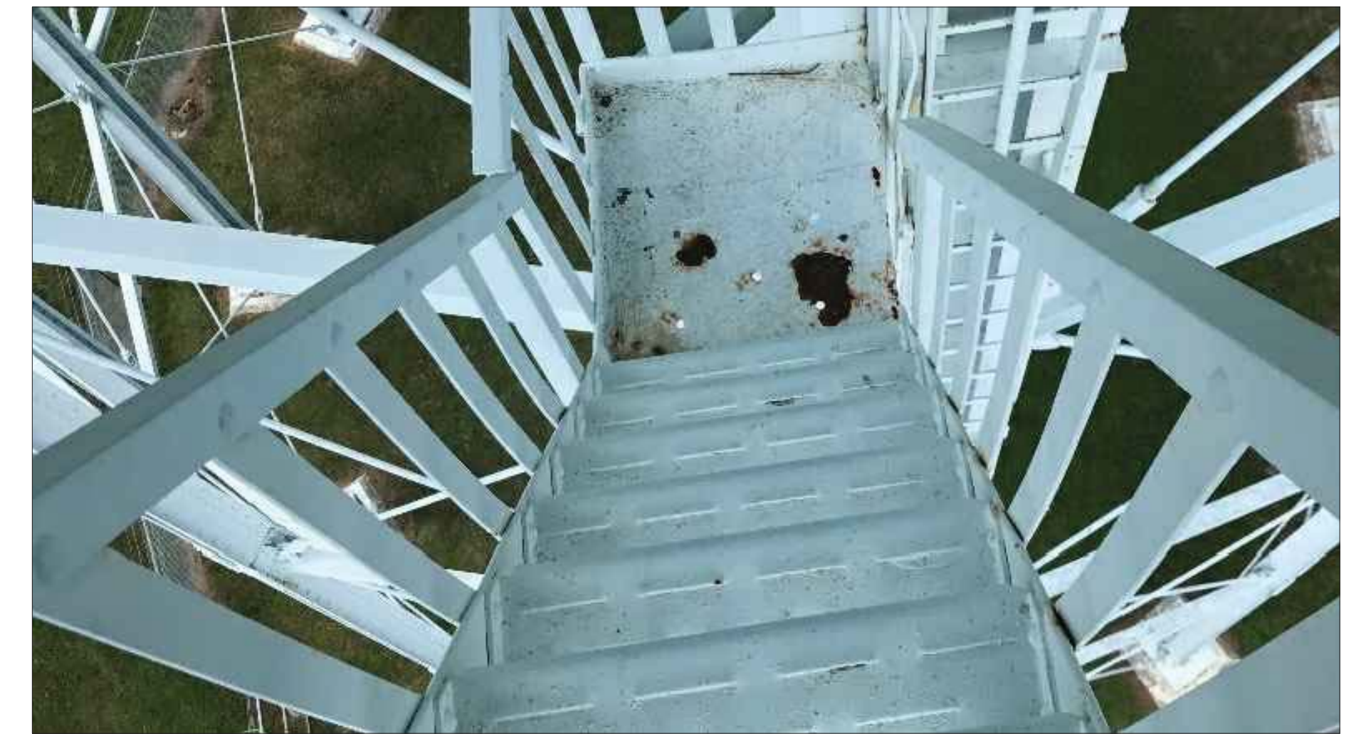
Figure 3. Stairs Leading from Landing at Top of Exterior Column-Mounted Ladder to Bowl Platform Repair corrosion at floor plate of landing.
