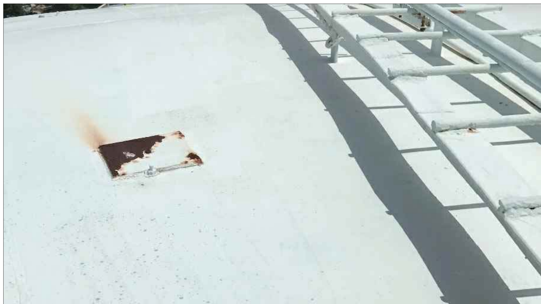
Figure 21. Cathodic Protection System Roof Plates on Top on Bowl Repair minor corrosion on cathodic protection system
