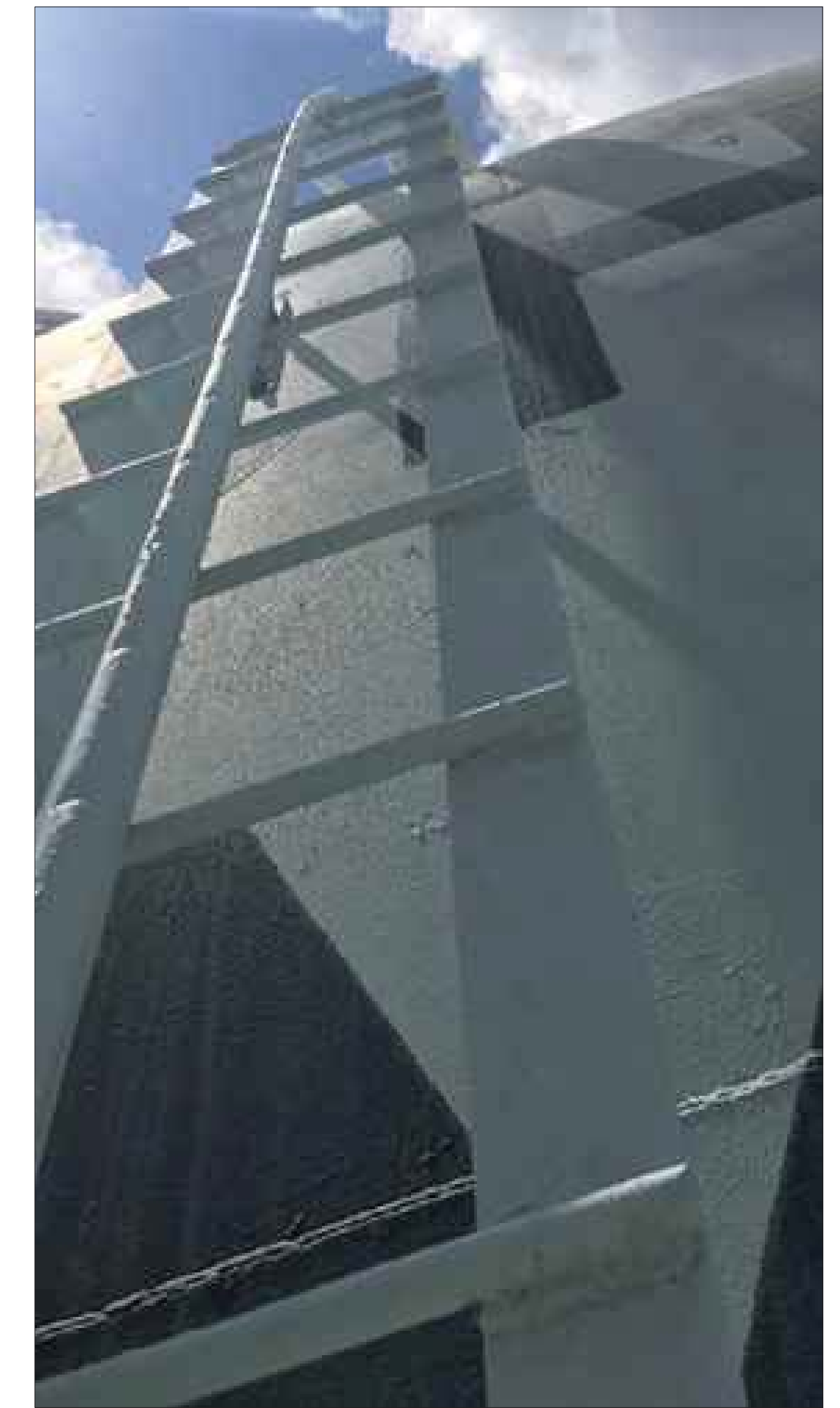
Figure 30. Exterior Ladder Leading to Top of Bowl Remove and replace exterior ladder
