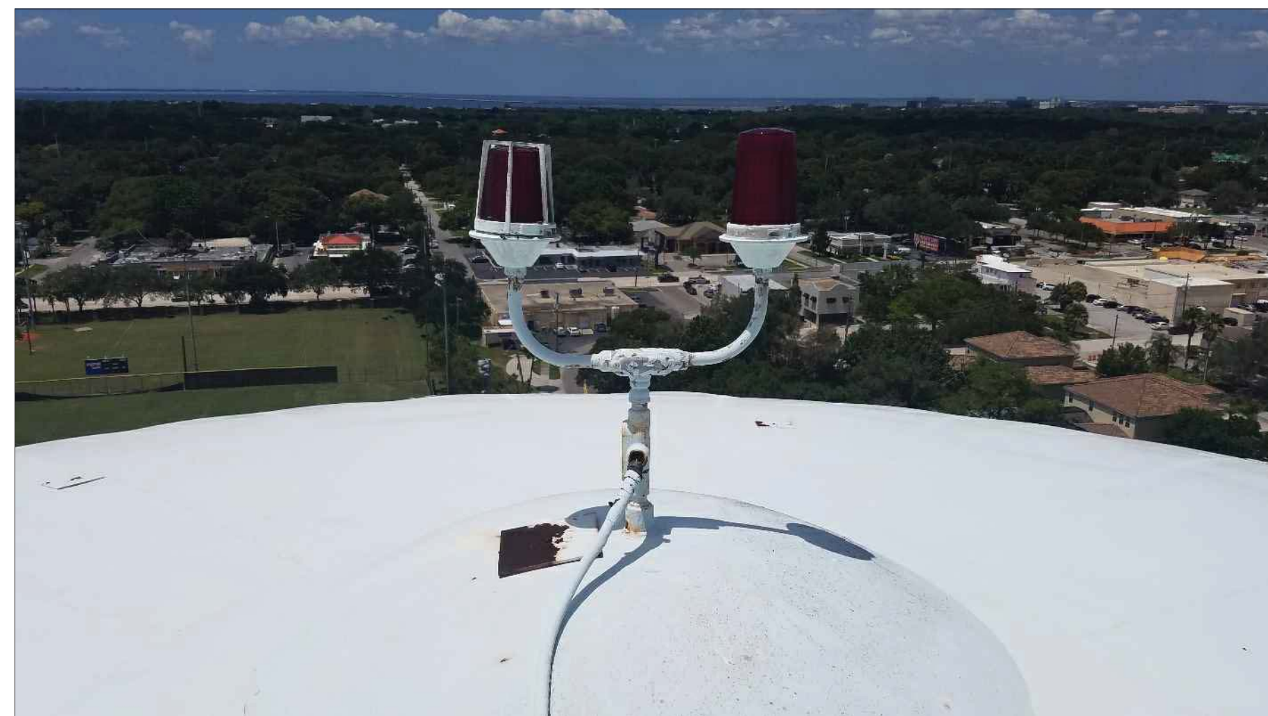
Figure 22. Aviation Lighting Repair minor corrosion peeling on aviation lighting
