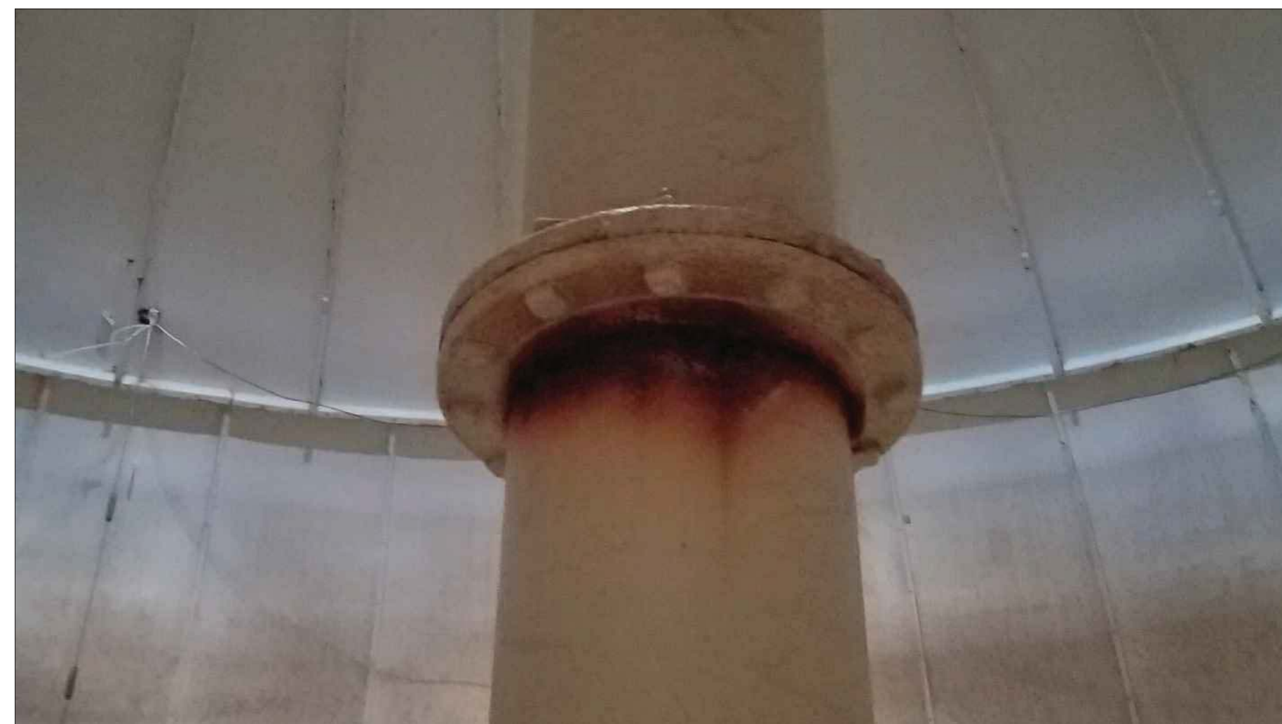
Figure 14. Bowl Interior Pipe Repair corrosion on influent pipe
