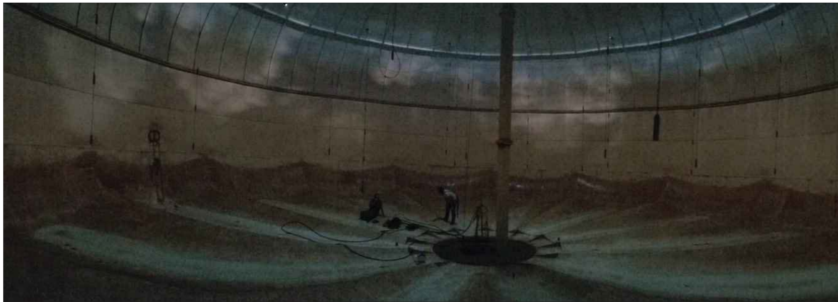
Figure 19. Interior Tank Bowl Provided for reference
