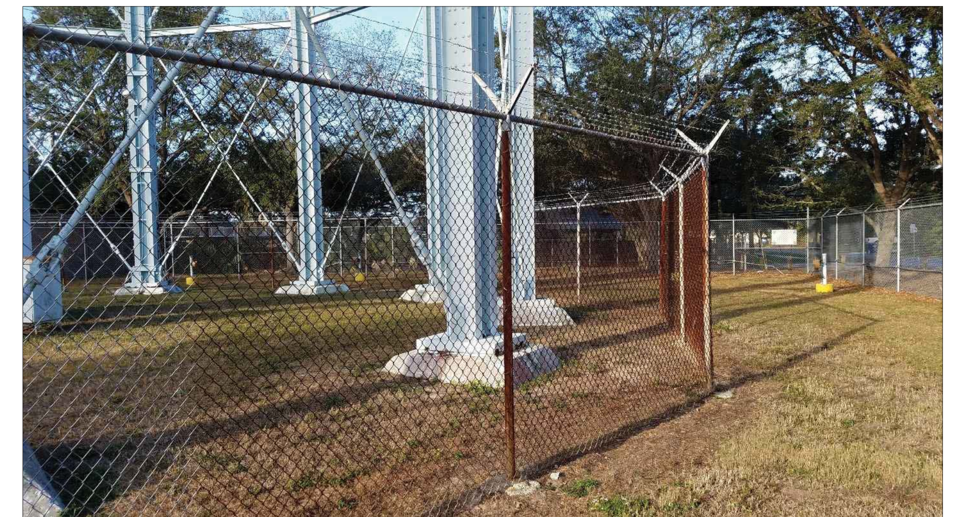
Figure 23. Exterior fence The exterior fence has corrosion on the support poles and chain link
