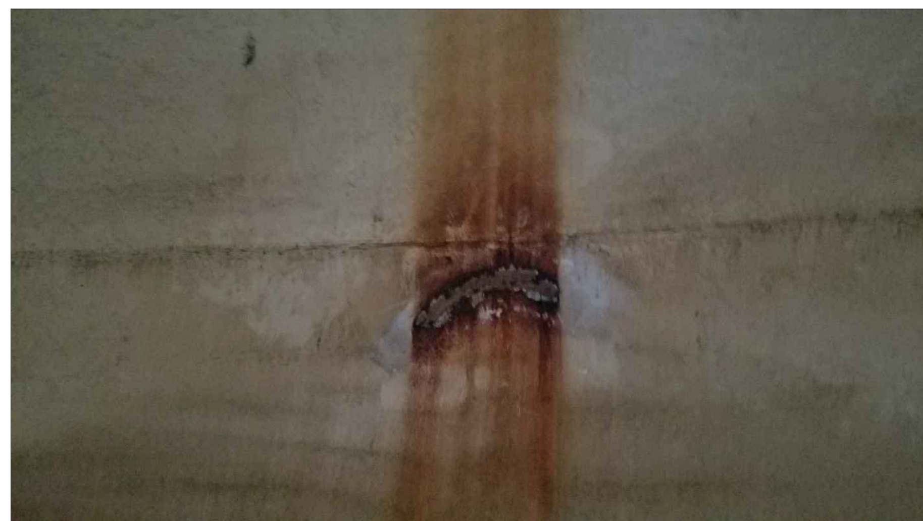
Figure 17. Tank Bowl Interior Repair pitted tank bowl as viewed from interior of the tank
