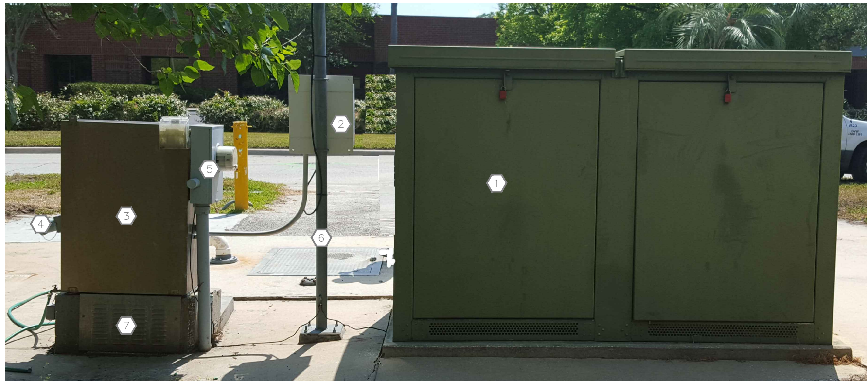
EXISTING CONTROL PANEL BACK VIEW
