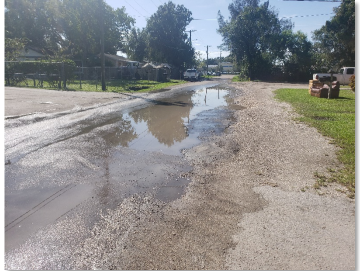
Figure 4.A: Image of Poor Road Condition
