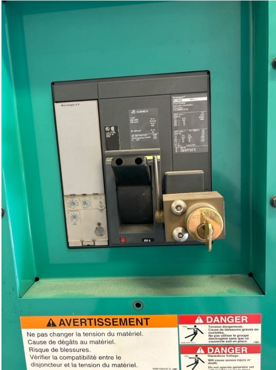
Controller in auto system ready
