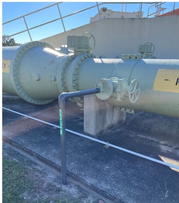
Figure 9 DLTWTF Pilot Raw Water Tap
