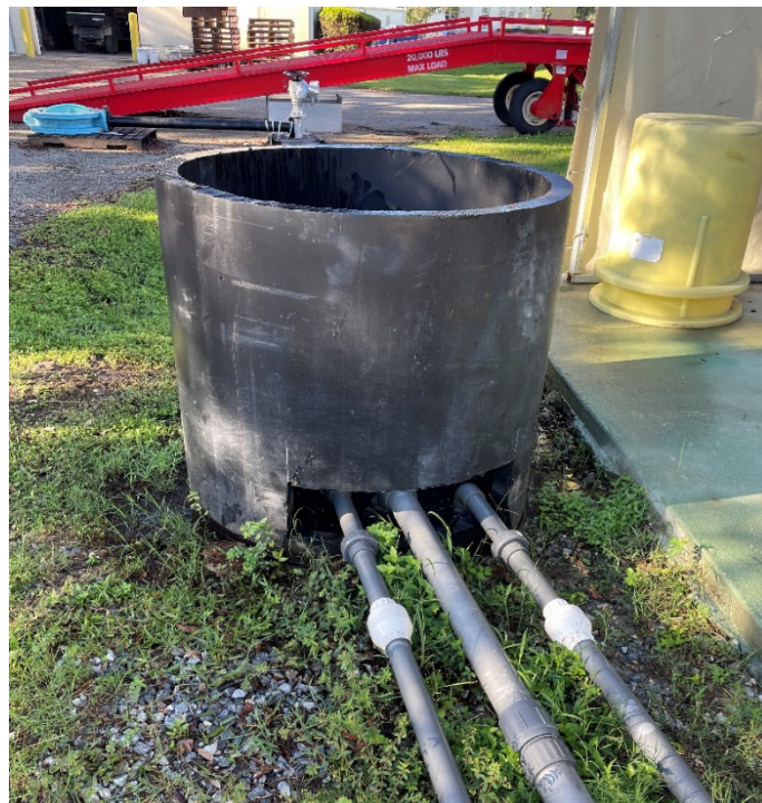
Figure 11 DLTWTF Pilot Waste/Overflow Collection Tank. Sump pumps sending water to Junction Box #4.
