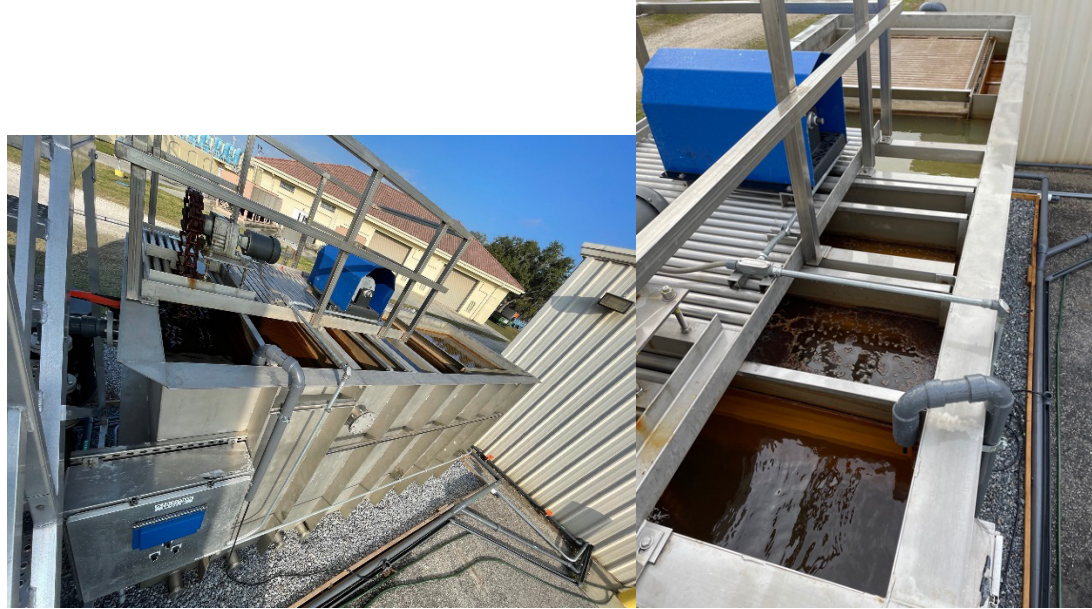
Figure 7 Pilot Floc/Sed Unit - S-side view (left) and top view (right).
