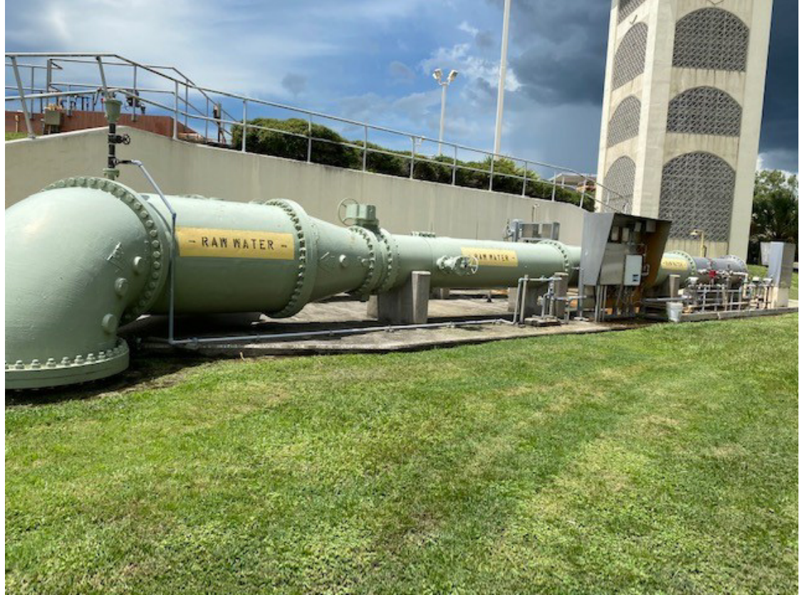
Figure 8 DLTWTF Actiflo® Piping
