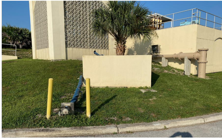
Figure 12 DLTWTF Junction Box #4
