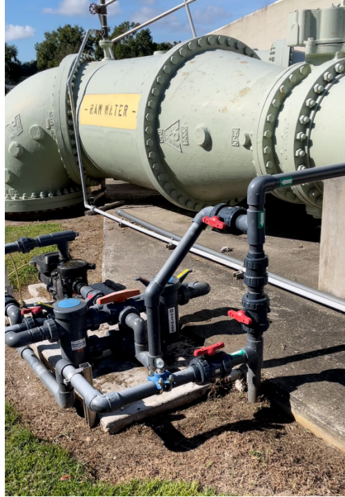
Figure 10 DLTWTF Pilot Raw Water Pump and Pre-filtration Setup
