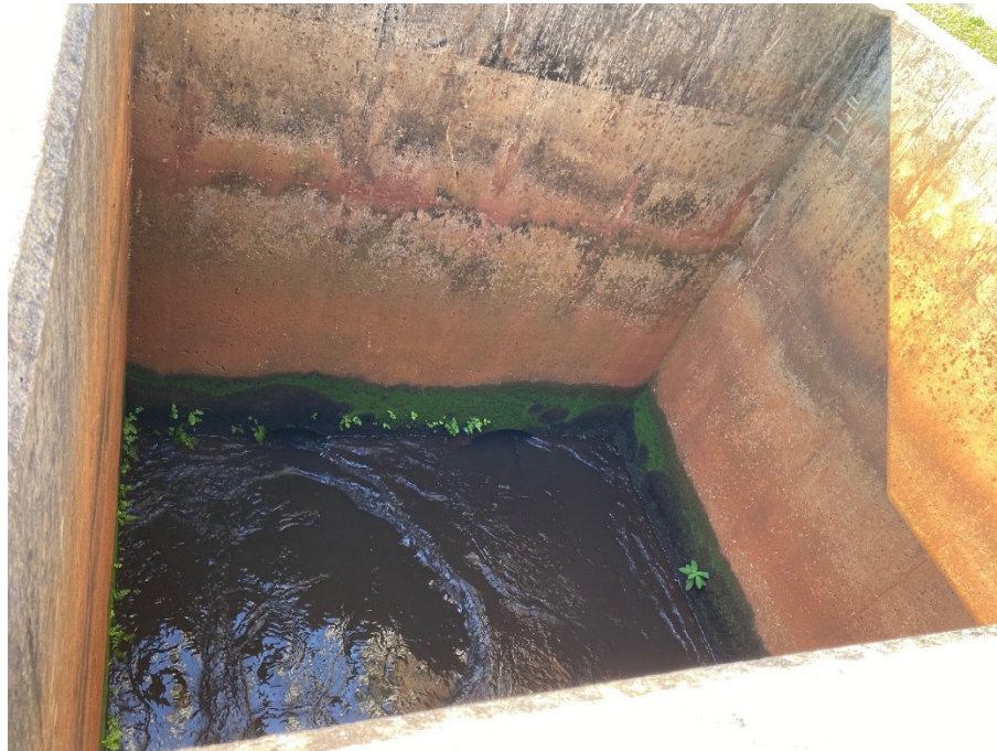
Figure 13 DLTWTF Junction Box #4 (internal)
