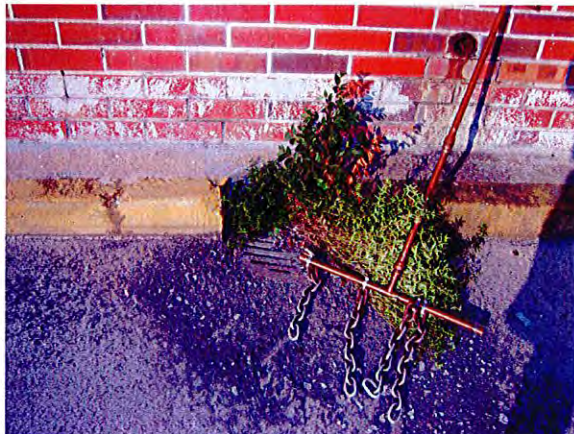
ACCUMULATED DEBRIS AND VEGETATION
