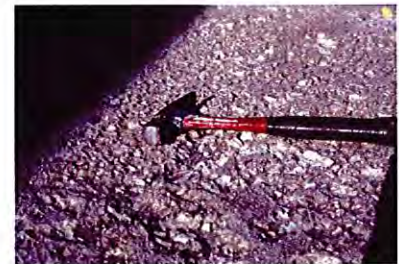
HEAVY SURFACE SCALING
