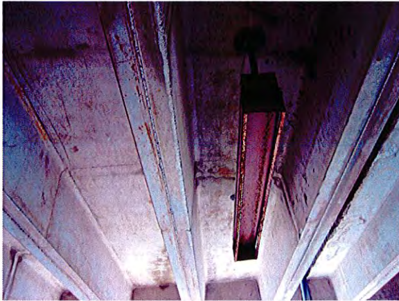
TYPICAL DEFECTIVE LIGHTING FIXTURE
