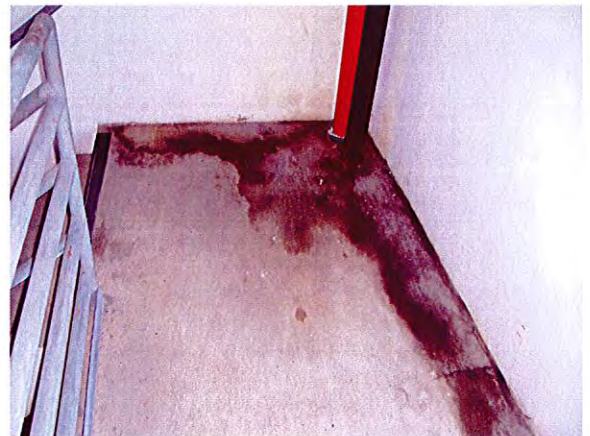
PONDING WATER @ STAIRTOWER LANDINGS
