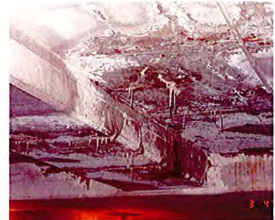
UNDERSIDE SLAB LEACHING
