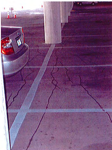
FLOOR SLAB CRACKING
