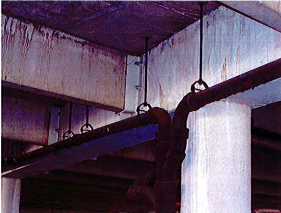
HEAVY CORROSION ON DRAIN PIPING
