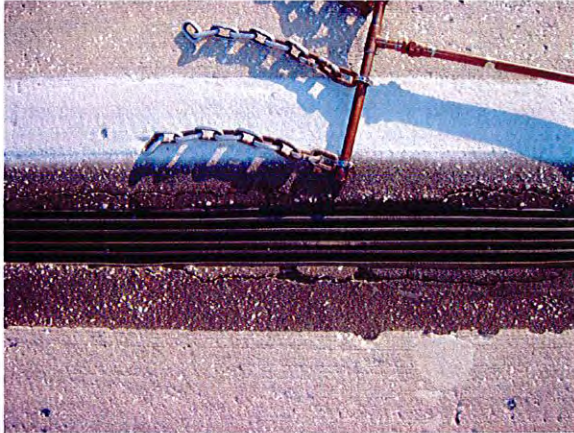
EXPANSION JOINT NOSING DETERIORATION
