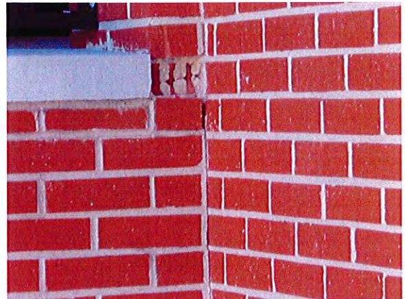
SPALLED BRICK FACE
