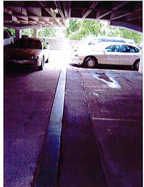
WASH AT EXPANSION JOINT
