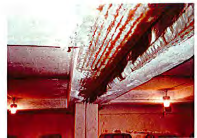
STEEL REINFORCEMENT RUSTING THROUGH CONCRETE BEAM
