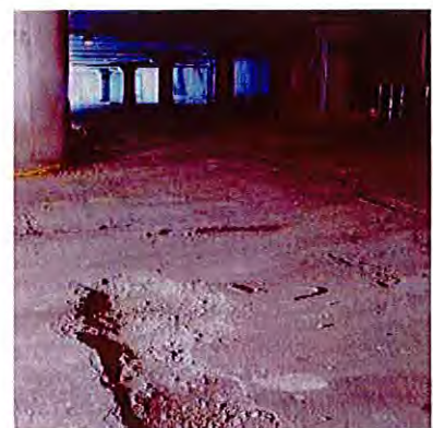
FLOOR SLAB SPALLING
