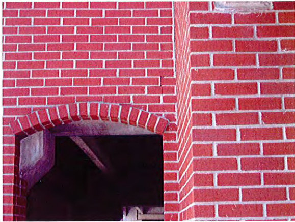
CRACKING @ MORTAR JOINTS
