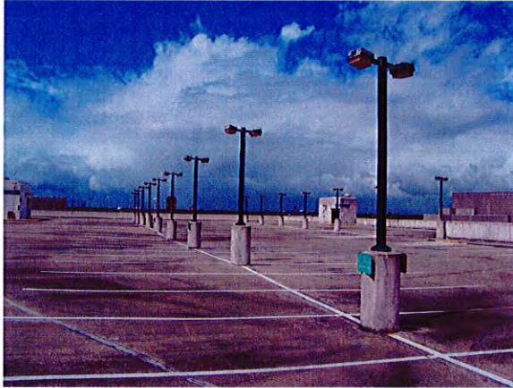
ROOF LEVEL POLE LIGHTS
