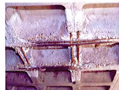
CONCRETE WAFFLE SLAB CORROSION
