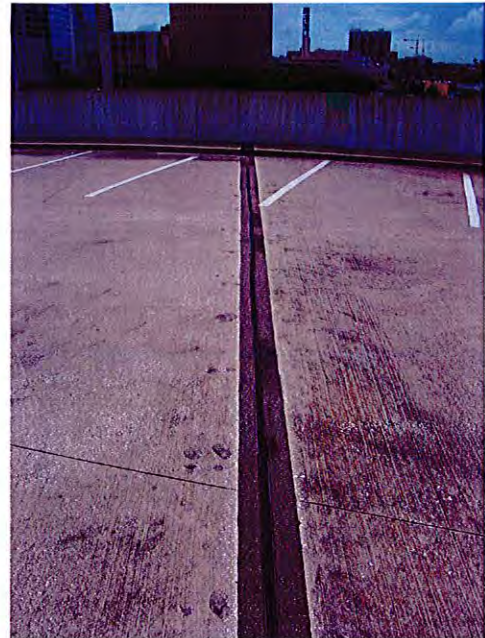
NEW EXPANSION JOINT
