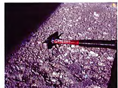
HEAVY SURFACE SCALING
