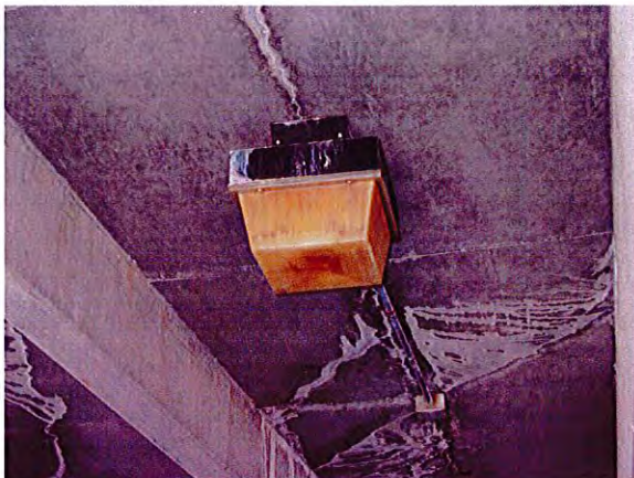
DISCOLORED LIGHT FIXTURE LENS
