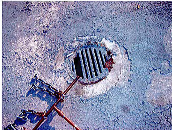
BROKEN DRAIN GRATE
