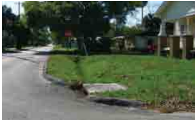
Stormwater conditions in East Ybor along 10th Avenue between 25 th and 26 th Streets.
